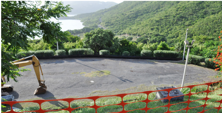
Heavy equipment prepare the grounds of the former overflow parking lot near the Social Sciences building on UVI's St. Thomas campus where a new 100-bed student residence facility will be built.
