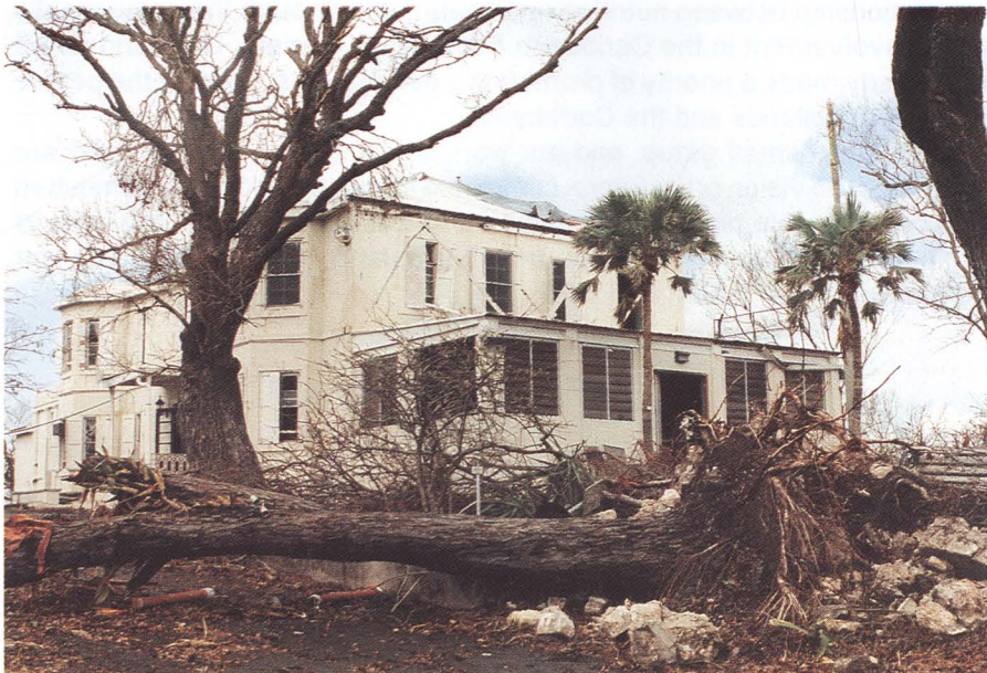
Top: Extension Great House Building in 1973. Bottom: Same building, just after Hurricane Hugo in 1989.
