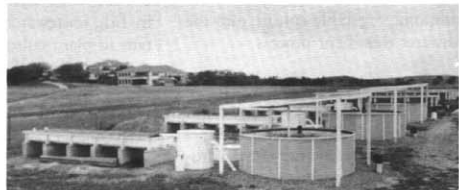
Completed tanks with hydroponic beds to the left.
